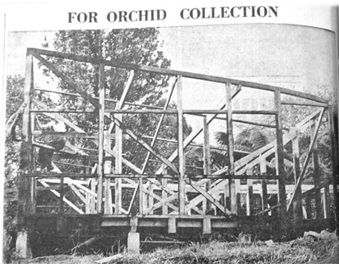
Shade house under construction for the Agnes Mary Parker memorial orchid collection. TDN , May 15, 1965.
