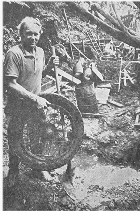
First job at the Waterwheel site is cleaning out the rubbish. Curator – George Fuller TH , April 2, 1974.
