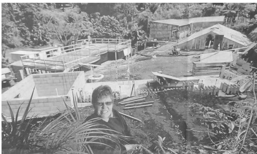
Stage three of the Fernery upgrade in progress. Fernery technical officer Donna Christiansen in the foreground. TDN , October 10, 2012.
