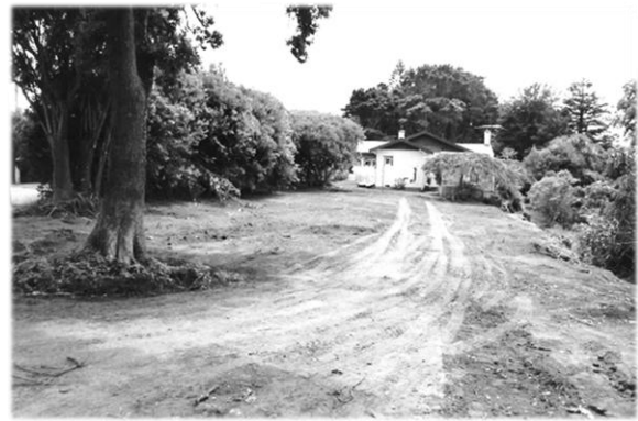
Victoria Road Car Park area during construction. Collection of NPDC. Parks Dept.
