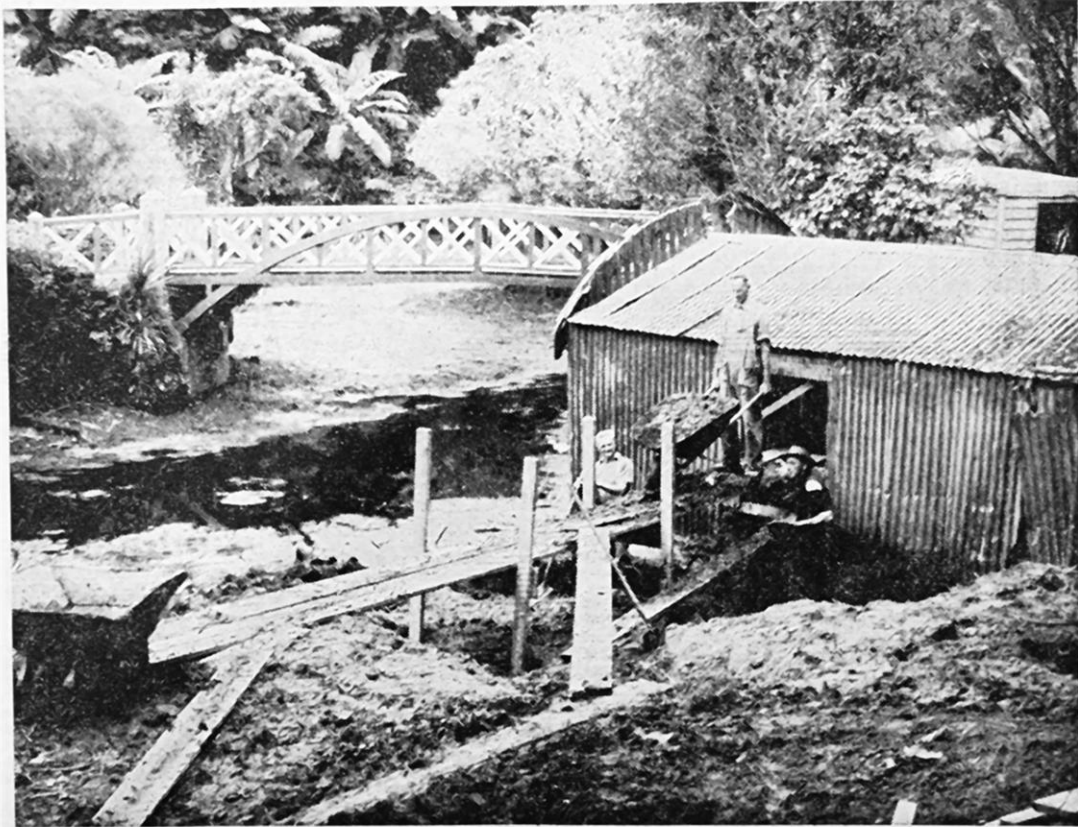
THE LEVEL of the main lake in Pukekura Park, New Plymouth, has been lowered about 4 feet 6 inches to allow work to begin on the site of the new boathouse. Members of the park staff are here seen removing soil from the area of the old boatshed. Some 220 cubic yards will have to be excavated before erection of the new building can begin. The upper, or boatshed, bridge is in the background.
