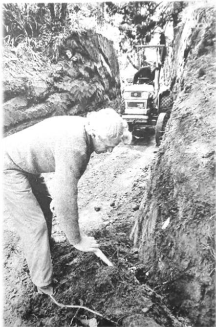
Bert Clark (left) and Ian Berry putting finishing touches to new path.
